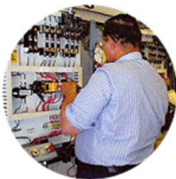
Understanding Low Voltage Electrical Systems
