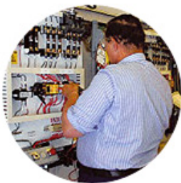
Understanding Low Voltage Electrical Systems
